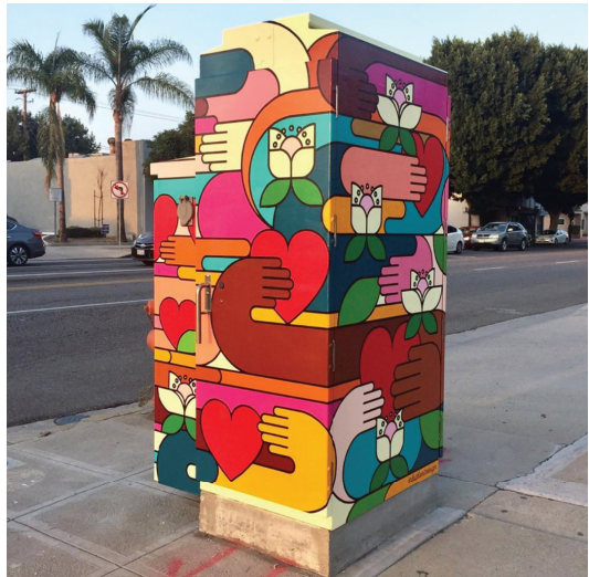
Electrical Box located at Buena Vista and Magnolia painted by Laishan Mui Ito and sponsored by Blast From The Past. (Photo by Ross A Benson)
